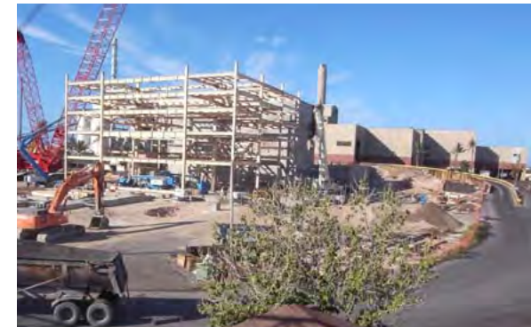
Construction of new Efw unit at HPOWER site in Honolulu in foreground. Existing units in background.
