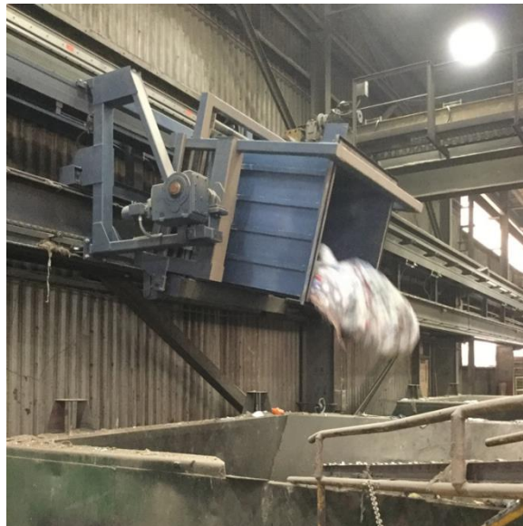
Figure 9 - WFS Dumping mechanism feeding MWC feed chute
