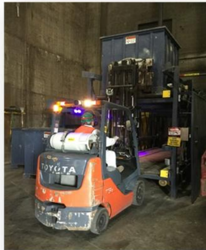
Figure 3.2.2 - WFS conveyors at tipping floor grade elevation. Example of forklift loading WFS Tipping Floor Supply Transfer conveyor.
